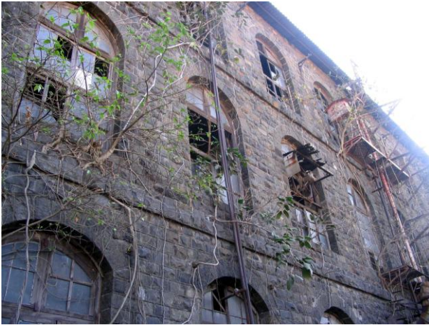
Tree growth on façade with windows in poor condition
