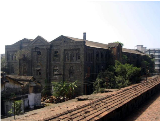
View of impressive stone façade of the Processing department with central triangular pediment
