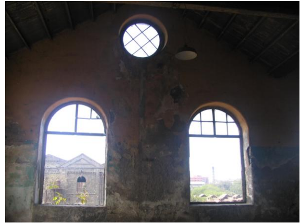
Plaster chipped off from the internal walls of the first floor
