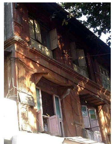
Front view of Rangari Badak Chawl no. 1 from N.M. Joshi road with window detail
