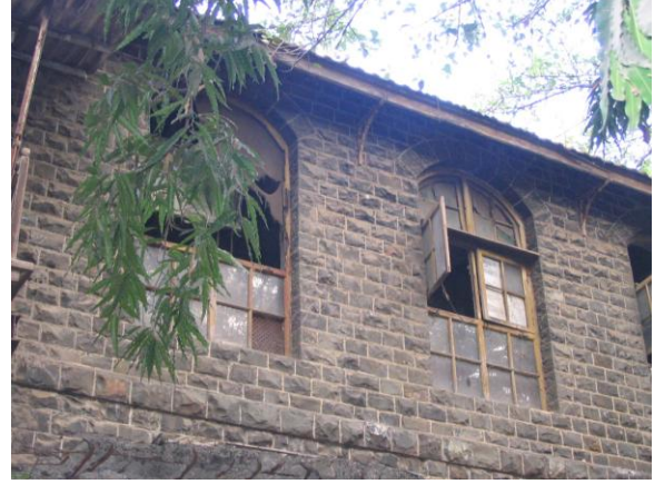
Part front view showing Black Basalt stone coursed masonry and segmental arched windows
