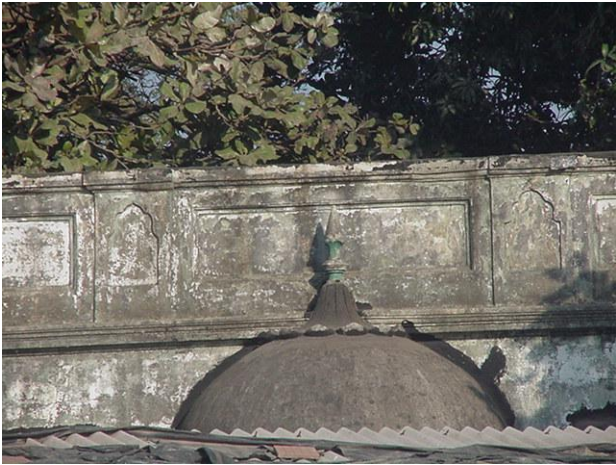
View of dome against compound wall of Bohara cemetery from Dr. E. Moses road.
