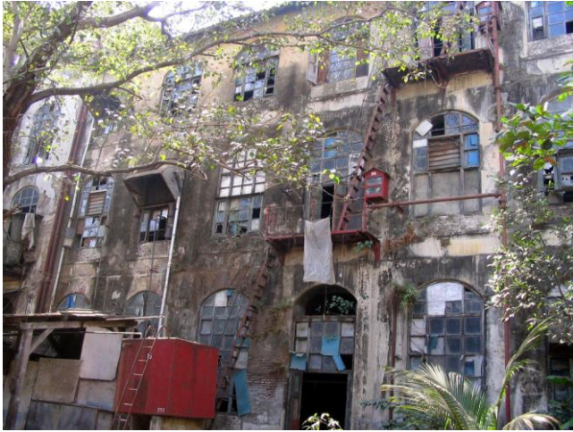
Plain façade with segmental arched windows showing weather attack and chipping of plaster
