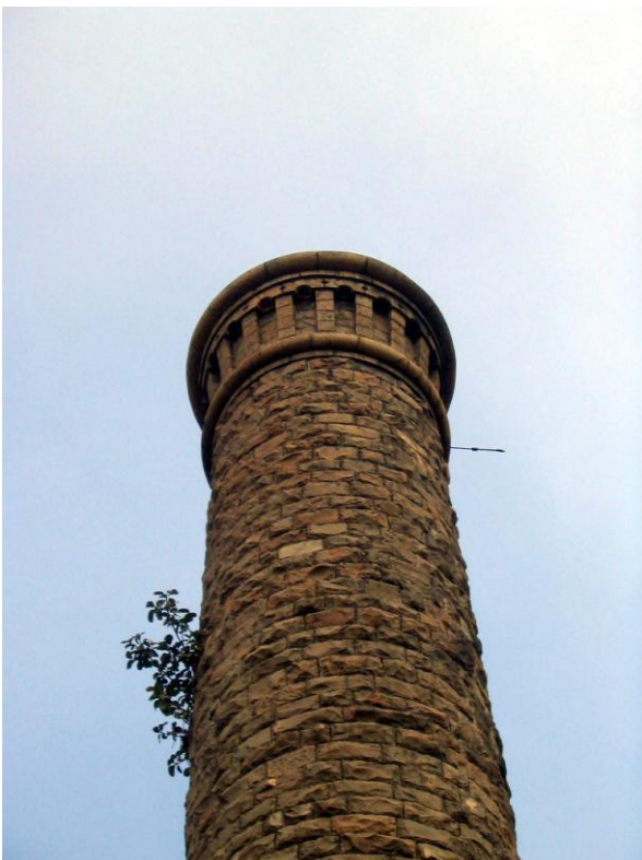
Horizontal ring bands & flutings in Black Basalt stone coursed masonry on top portion of chimney
