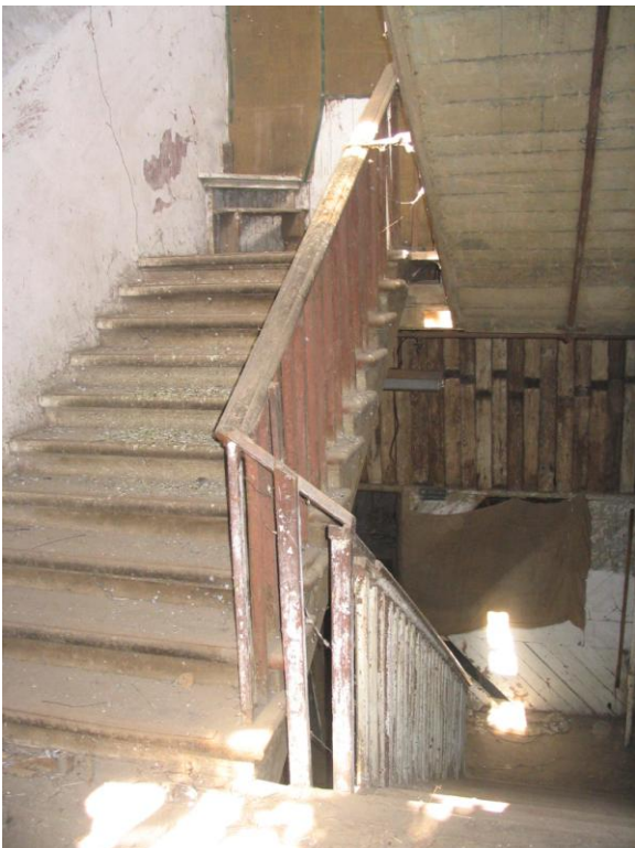
Dog legged wooden staircase
