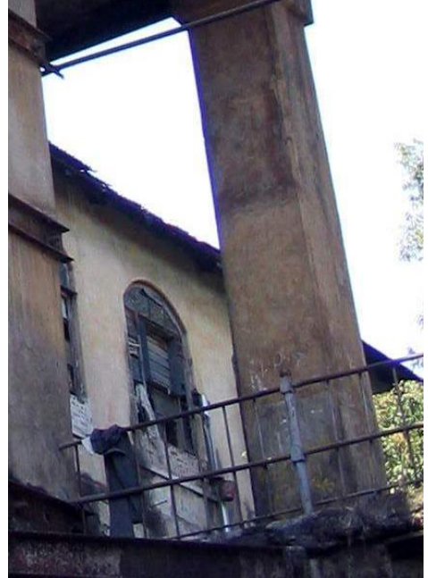
Windows and railing in dilapidated state
