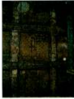
Reinforcement of coffered slab exposed after removal of loose concrete cover.
