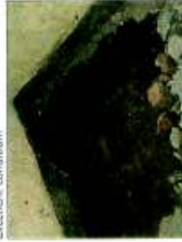
Shalhad stone flooring explored in the rooms was fairly damaged and uneven.
