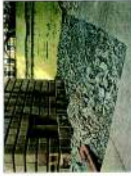
Layer of P.C.C. and murrum around the structure was much deeper than estimated.
