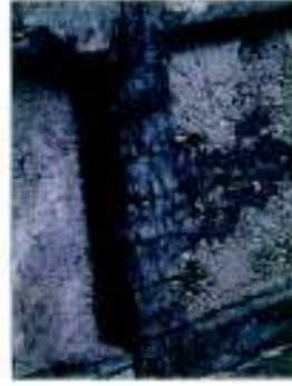
Application of Polymer modified plaster after introduction of additional reinforcement and new stirrups
