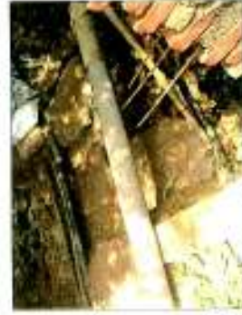
Organisation of the HT and LT cable network of was a challenging task
