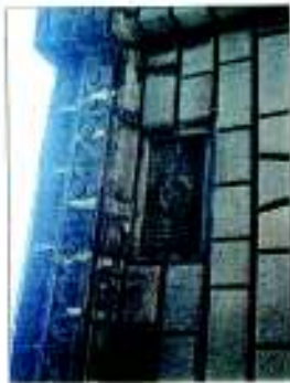
Decorative façade features demystified by soiling / tar stains and cement application (before restoration)
