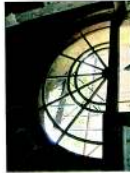
Stain bars in the semi-circular portion of the arched opening placed in position.
