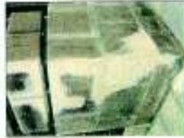
Plastic Repairs using lime mortar in locations where part stones had spalled
