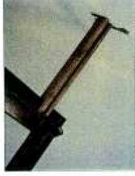
Wooden frame suspended from slab with GI link chains to install lighting fixtures
