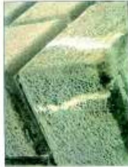
Damaged corner stone restored by stitching with SS pins and lime mortar jointing.
