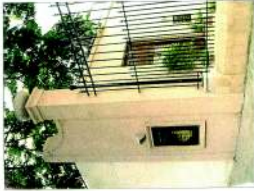
Junction of old and new security walls sensitively treated to achieve a subtle transition. A Brass Plaque with a key map of Ballard Estate area is aptly placed here.
