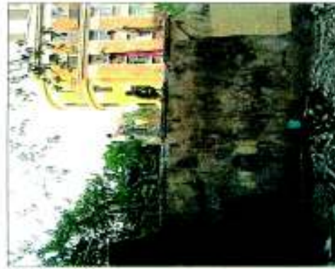
Layers of loose filling material revealed after removal of tar felt.
