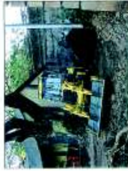
Removal of debris between the structure and the tree after demolition of the shed
