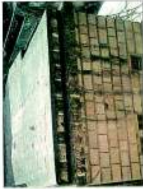
FACADE SOILED WITH STAINS (DUE TO WEATHERING AND TAR FROM THE TAR FELT ROOF PROTECTION) BEFORE RESTORATION
