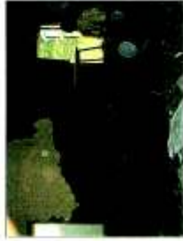
Removal of plaster exposes the composite masonry (Stone masonry with brick leaf wall)
