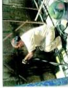
An attempt at use of pressurised steam to remove stubborn tar stains from the stone surface did not prove effective.
