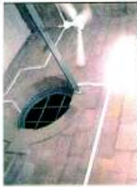
SENSITIVE DESIGN AND LAYOUT OF ELECTRICAL WIRING AND FITTINGS - BEFORE RESTORATION
