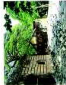
Security wall demolished to offer visibility to the structure and to re-establish the image of the node
