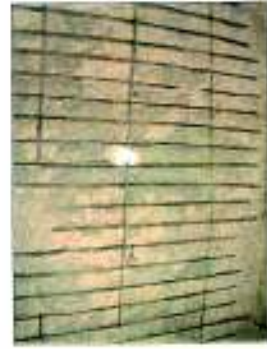
Reinforcement of slab exposed after removal of loose concrete cover
