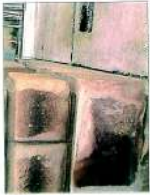
NETWORK OF SERVICES AROUND THE STRUCTURE LACKED ORGANISATION - BEFORE RESTORATION
