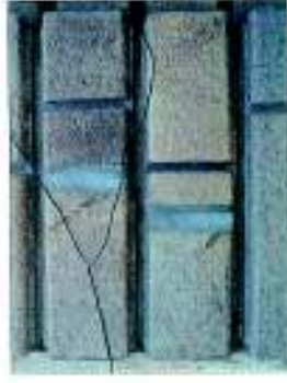
Deep recessed joints in stone masonry filled with cement mortar (before restoration)
