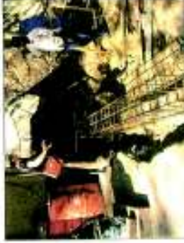
R.C.C. Beams laid across the massive tree roots to support the masonry above
