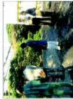
Inspection of roof slab before removal of the layer of tar felt.
