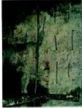
Vertical structural crack in the masonry wall between the central hall and the rooms stitched with SS pins.
