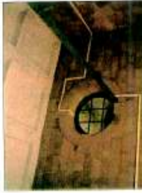
OX EYE WINDOW BEFORE RESTORATION
