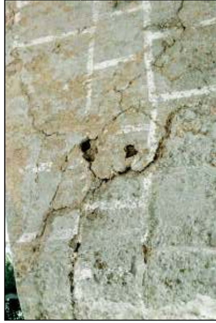
Condition prior restoration – accretions of cement plaster
