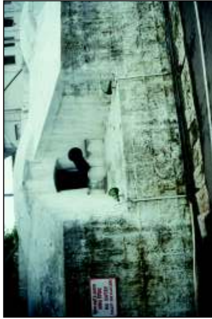
Condition prior restoration – accretions of cement paint
