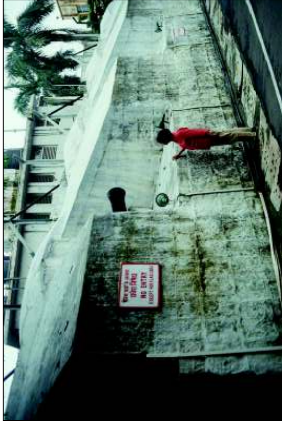
Security fencing in steel angles & mesh was mounted onto the Fort wall directly. This has been cleared and the walls restored.
