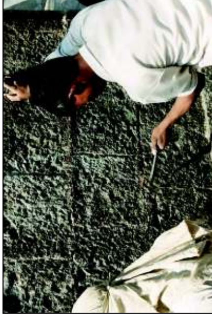
Removal of cementitious accretions by gentle tapping & soft brushing of pre-wetted stone surfaces
