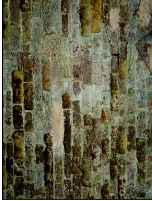
Condition of Laterite stones exposed after removal of paint & cement plaster
