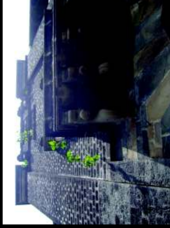
Photographs showing Peepal plants growing out of masonry joints along sections of deteriorated pointing, specially where there is a source of water leakage close by as a result of choked drainage outlets, leaking rain water down takes or air conditioner units
