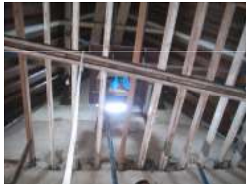
Repair to ends of timber joists.
