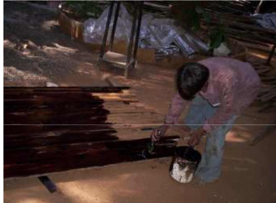
All timber New, or old was treated with solignum before polishing. All Malaysian sal was treated with linseed oil coating.
