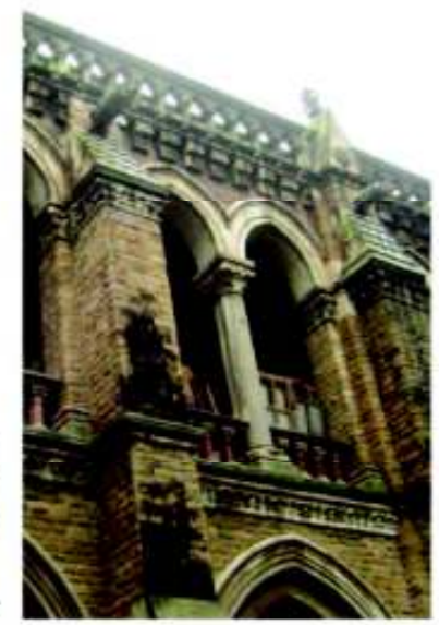
6 Staining of Stone masonry
