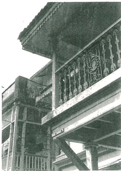
Above Koli Housing in Salsette Below Victorian Motif on Railing Source – Joshi (1995)
