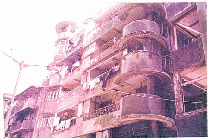
Building Condition Fair to Poor Source RCACC 1999 / 2000
