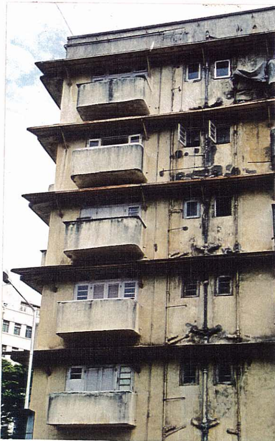
Deteriorating Condition of the building Façade (Moonlight)
