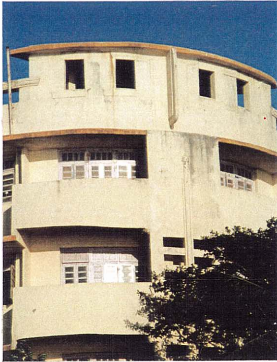
Alterations: - Grooves Lost Due to Replastering. (Riveira)
