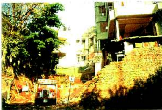
"Shree Sadan" - Residence of the Dahanukars. The original plot has been sub-divided, original bungalow demolished and built over with New building
