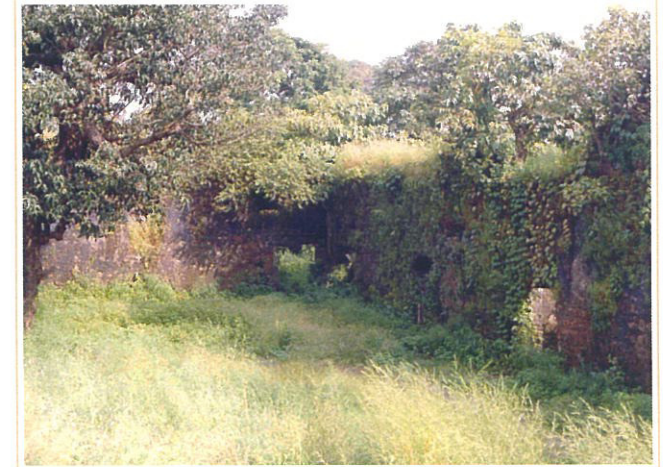
Excessive overgrown vegetation leading to the deterioration of the fort
