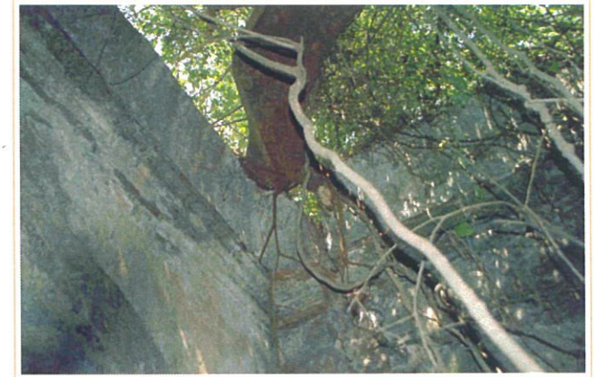
Remains of a flat-topped vault in one of the rooms in the fort
