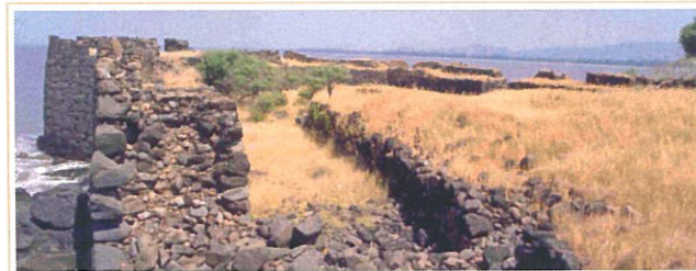
Ruinous state of the ramparts and the bastions.
