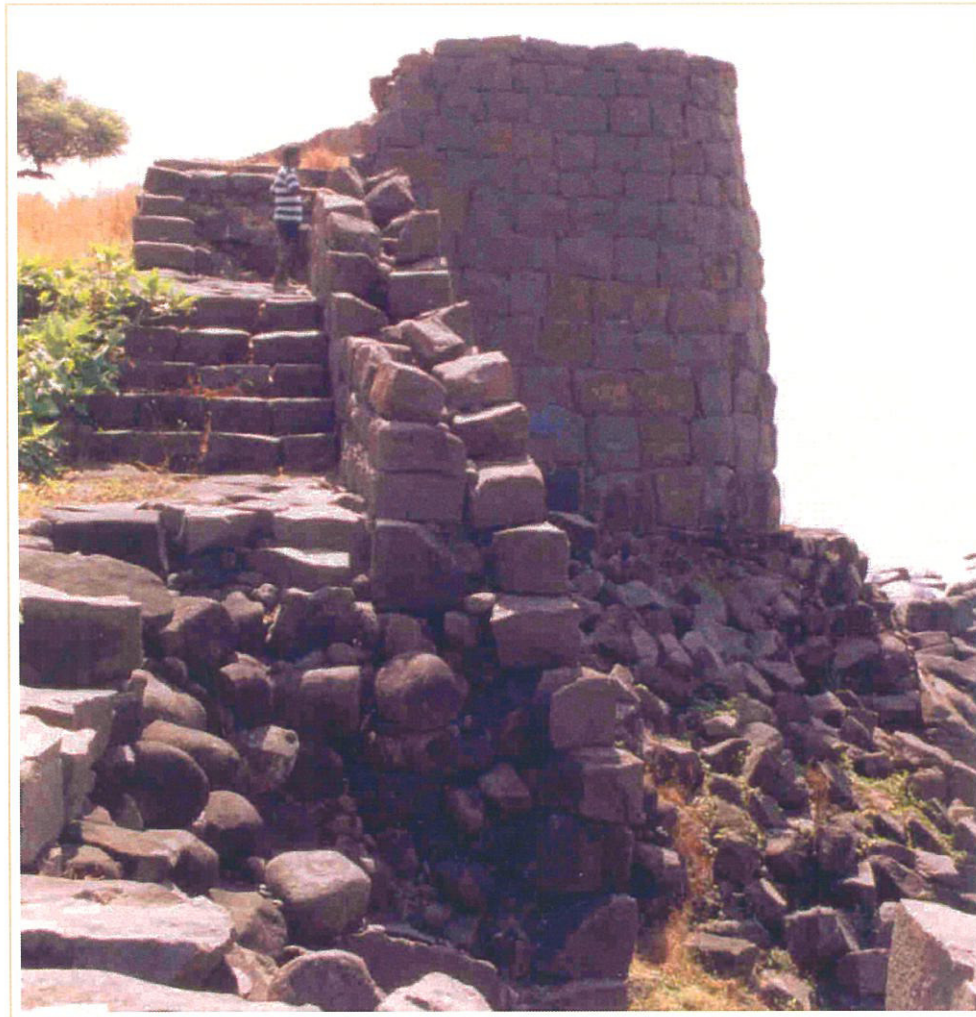
Collapsed portion of steps leading to the bastion
