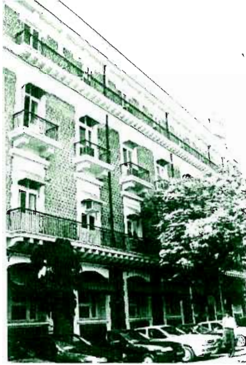
The grand hotel has painted some of its stone, given a protective coat to stone and done re-pointing using epoxy/m seal which is detrimental to fabric.
