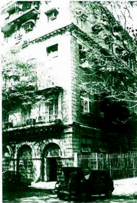
Insensitive placement of AC enclosed within box window completely ruins the esthetic character. Box grills like this should be removed and in future should not be allowed.
