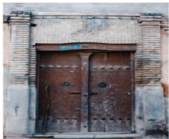
Damages due to ascending moisture
