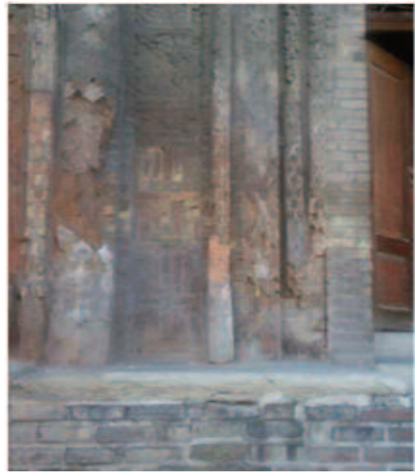
Penetration of moisture into the pores of the buildings and freezing between the bricks which shatters them in cold region
