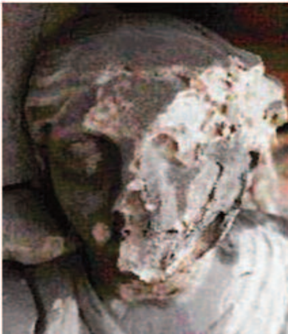
Exhibits shows decay typical of magnesian limestone by salt crystallisation in a polluted urban environment.
