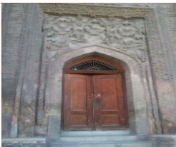
Moisture along with fluctuations in temperature leads to disintegration of the façade
