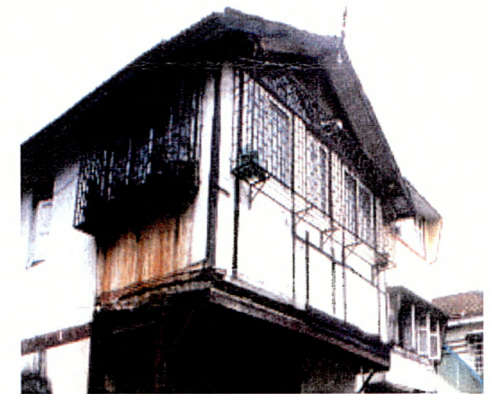
Box grills mar the façade and the precinct's character
