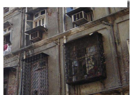
SERVICES IN BAD CONDITION
