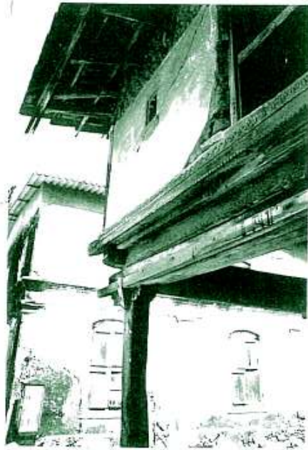
Trabeated timber-framed structure in dilapidated condition, Manori Source: RCACC (2002)
